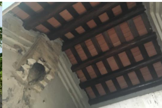
Fig 46. Site photos showing the remaining chimney in the Servants' Quarters (interior), 2016 (Source: Photo took by Betty Tay)
