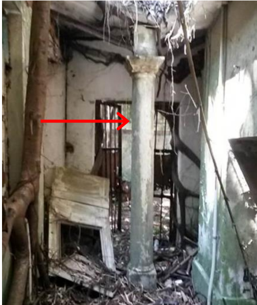
Fig 47. Site photo showing the column of the covered walkway, 2013 (Source: Revitalising Historic Buildings Through Partnership Scheme – Old Dairy Farm Senior Staff Quarters – Resource Kit, 2013, P.75)
