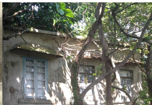
Fig 42. Site photo showing the flat roof structure, 2013 (Source: Photo took by Betty Tay)
