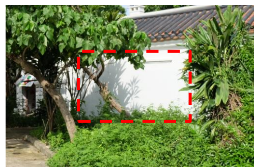
Fig 50. Site photo showing the windows had been blocked with original moulded canopies, 2016 (Source: Photo taken by Betty Tay)
