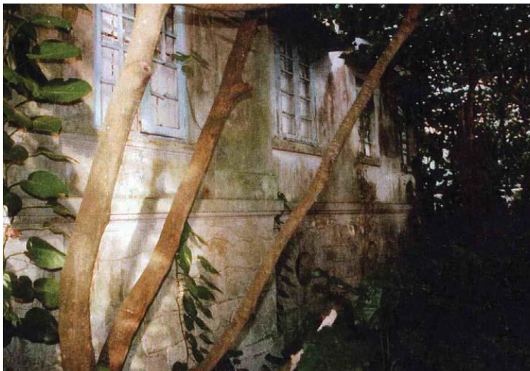
Fig 52. View of the SSQ before the basic repair works carried out by ArchSD. Year of photo taken is unknown. (Source: Antiquities and Monuments Office, Hong Kong)
