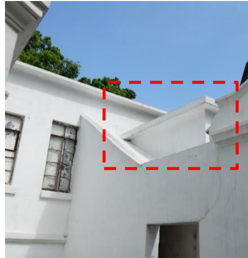
Fig 40. Site photo showing the flat roof structure attached to the Main Building, 2016 (Source: Photo took by Betty Tay)
