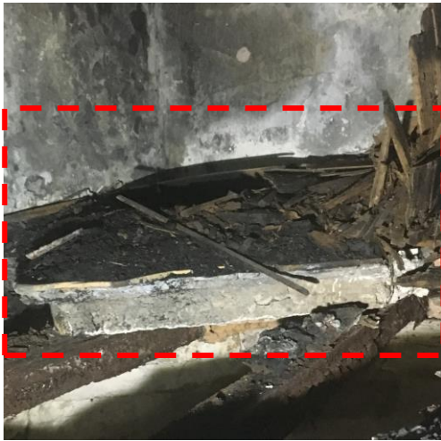
Fig 30. Site photo showing the plinth of the fire place, 2016 (Source: Photo took by Betty Tay)
