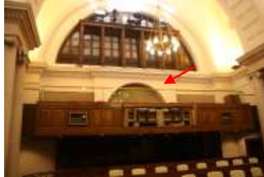
The north public gallery later added. The original arched moulding is still visible
