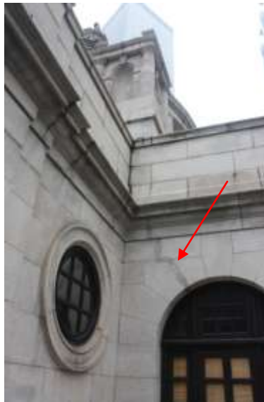
Fig. 23 Cracks developed on various locations on the building which led to the temporary closure of the entire building in 1978 for restoration. The photo shows one of the cracks located on the granite surface in 2/F under the central dome being repaired in 1980s. (Pointed)
