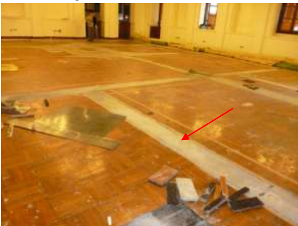
The square-patterned timber strip flooring finish reviewed after the removal of carpets. Trunk damages are discovered. (pointed)
