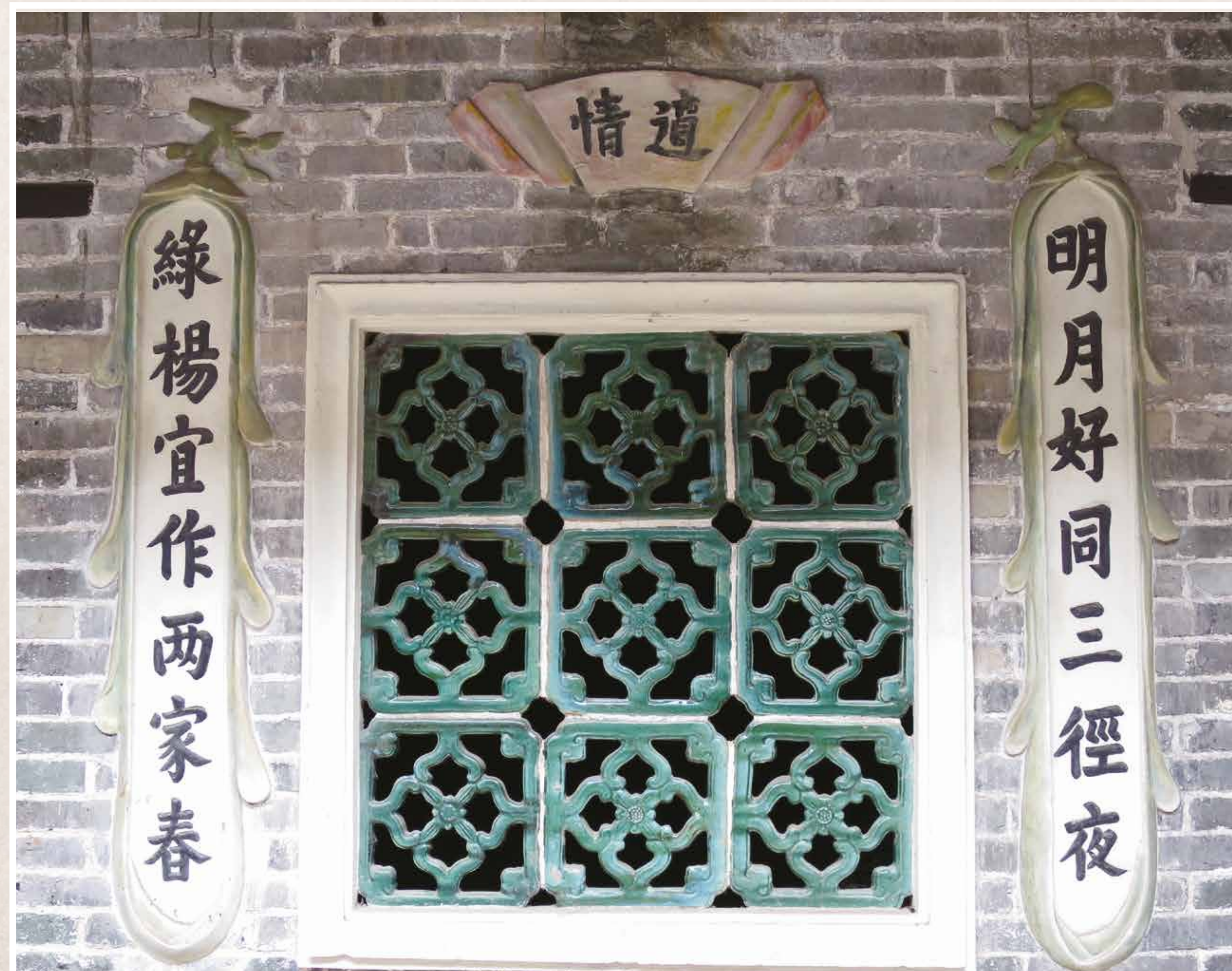
綠色琉璃陶製漏窗及灰塑對聯 Green glazed ceramic grilles flanked by a pair of plaster couplets on the ground floor of the front block
